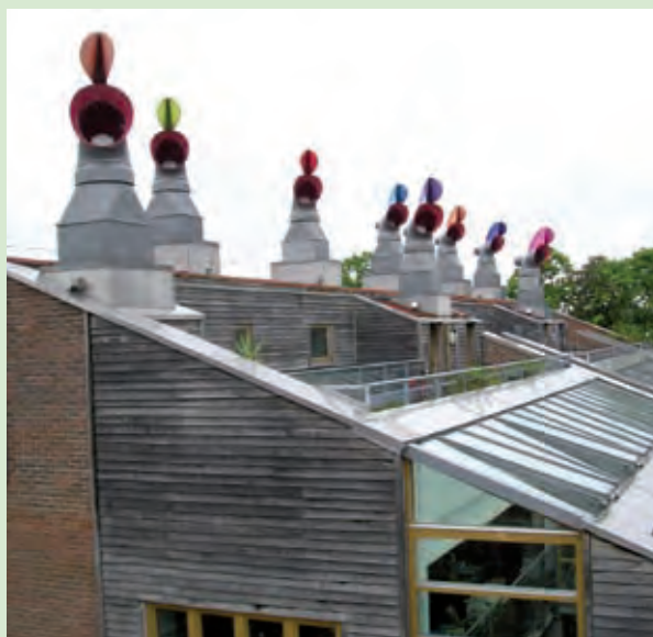
Passive stack ventilation, BedZED development of homes, community facilities and workspace at Wallington, South London
