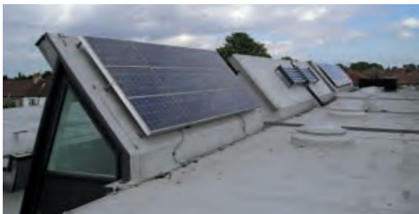
Photovoltaics and solar panel Upland Primary School, Bexleyheath
