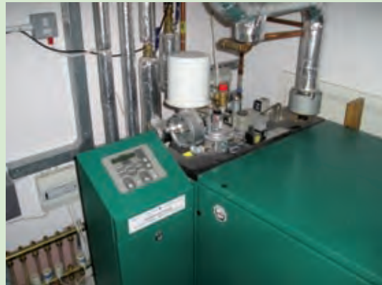
Efficient combined heat and power plant
