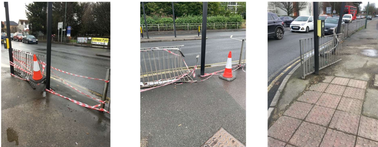
Figure 2 - Street Furniture Damage – Central Refuge Damage/Missing Barriers
