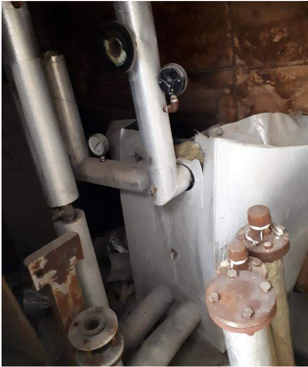
Figure 11: Previous DH plant
