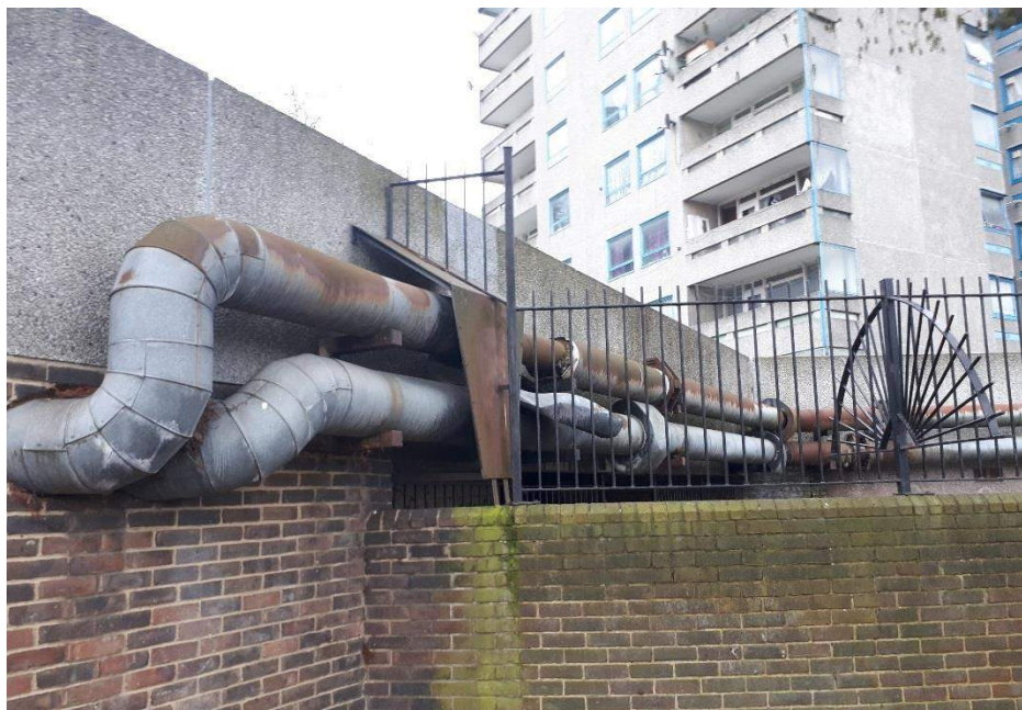
Figure 25: Example of above-ground DH pipework, mounted on side of Parkview Estate podium walkway
