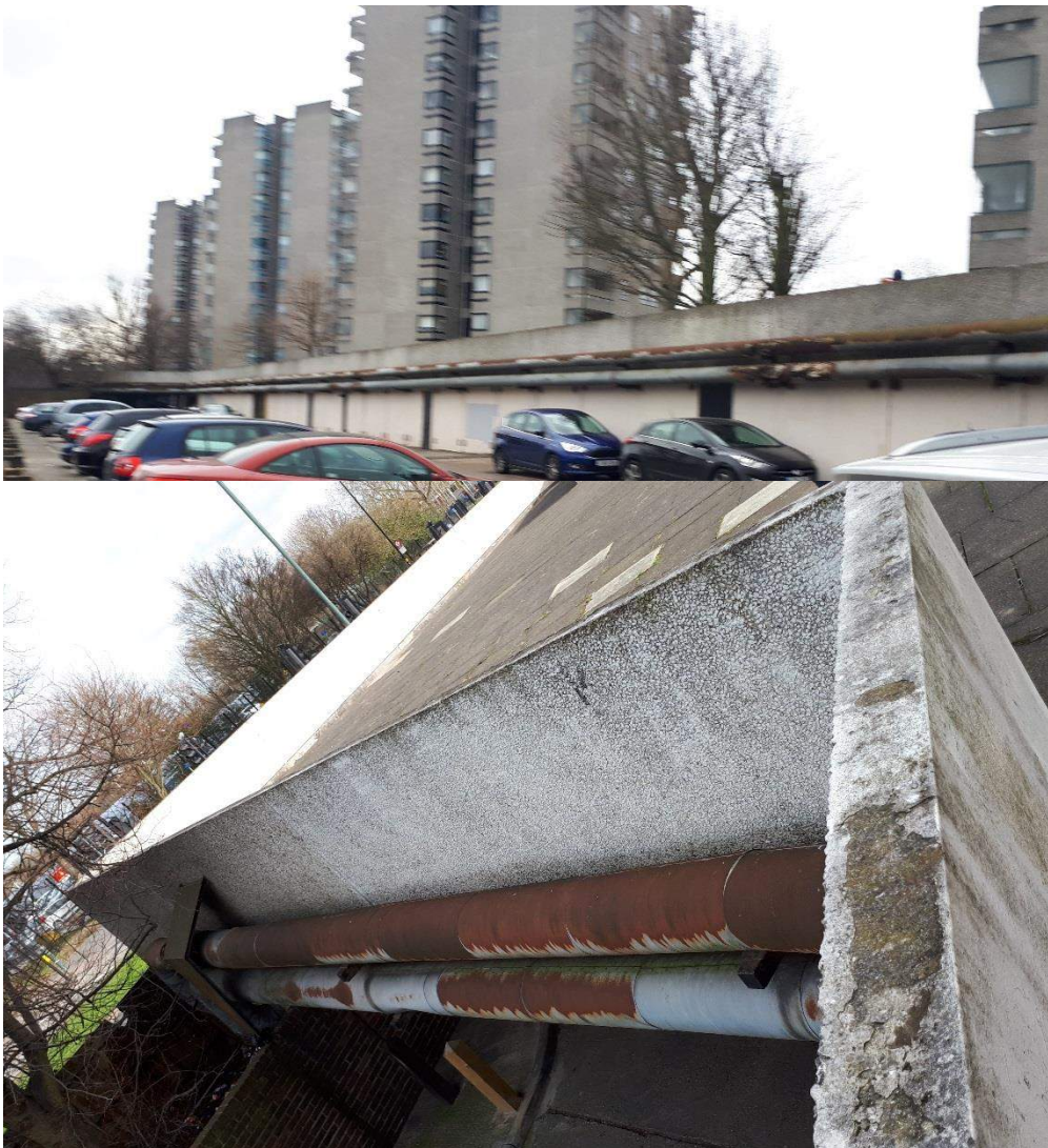
Figure 14: Examples of above-ground defunct DH pipework
