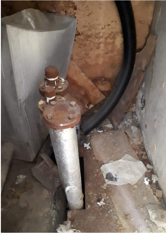
Figure 10: Capped DH pipework entering Osney House
