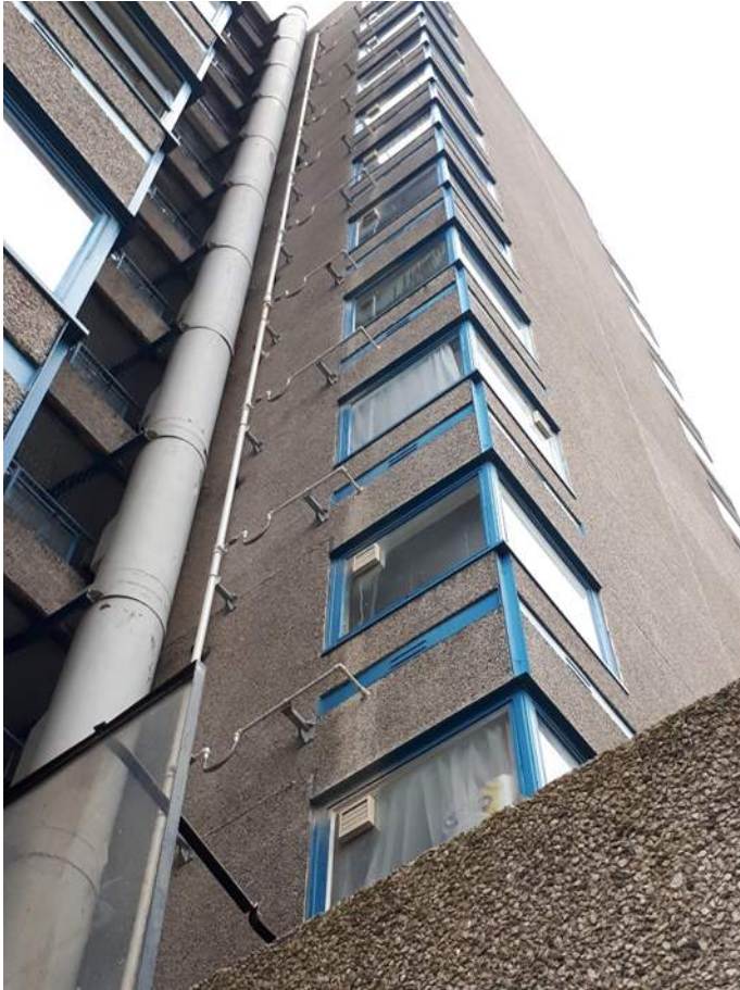
Figure 6: Visible external gas distribution pipework to individual flats
